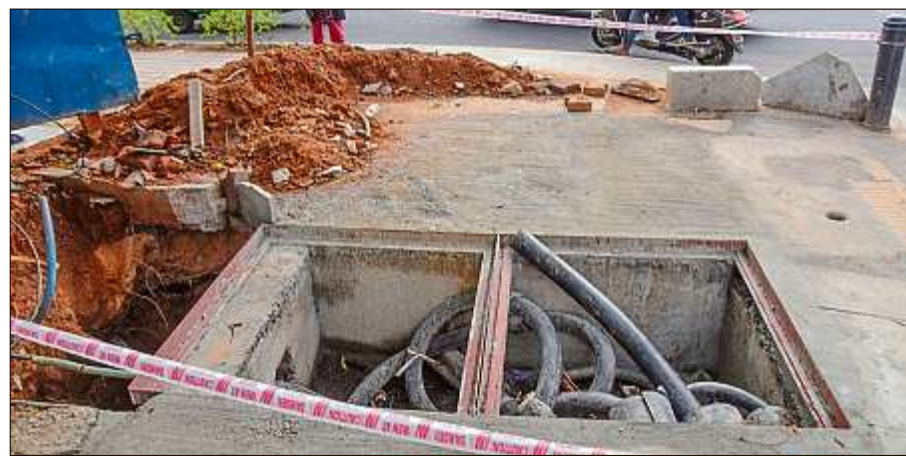
Slabs seen removed along Church Street, causing inconvenience to pedestrians, on Friday.
